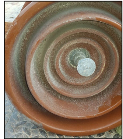
Contamination on insulator (above)
